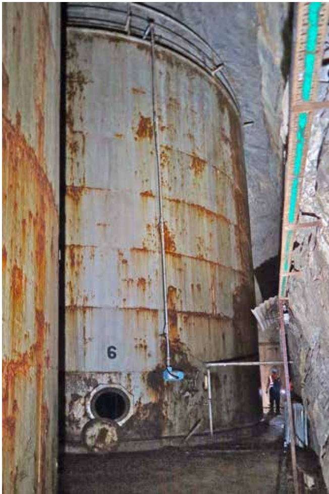
Project C: two of the series of petrol storage tanks. Photo Clive Penfold
